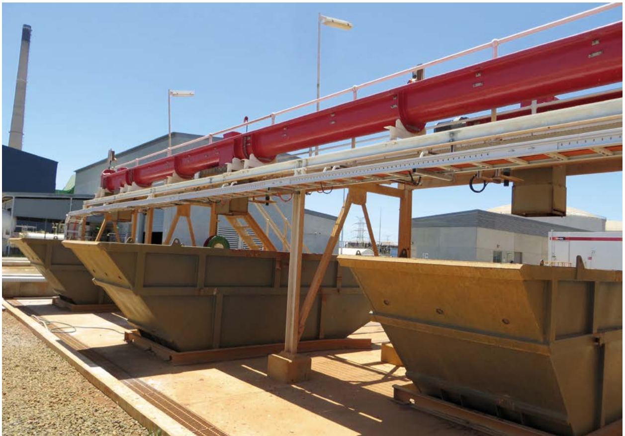
Water treatment: desalination plant
