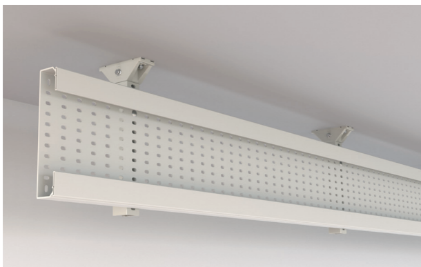
Pendant support for cable tray
