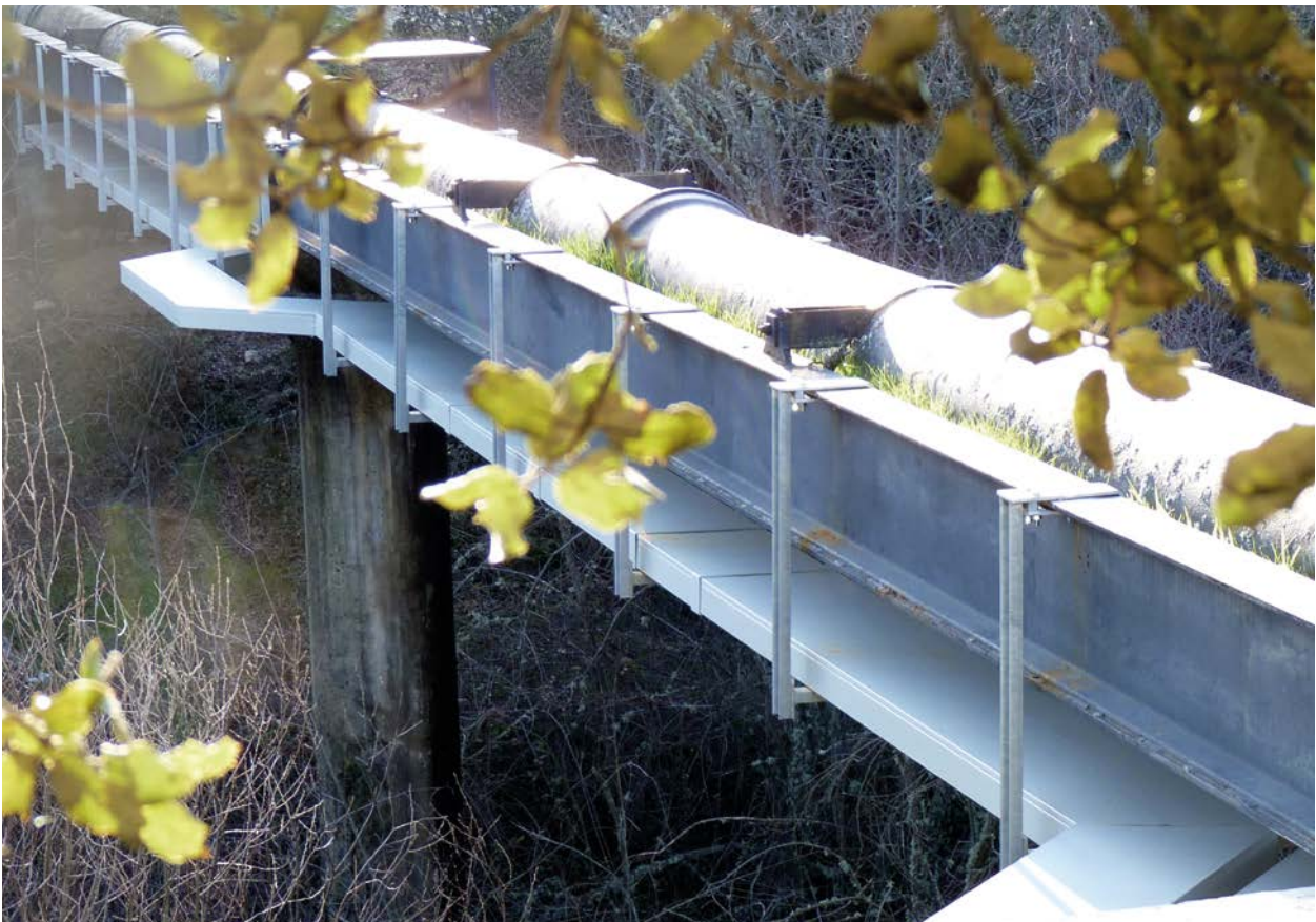
Power generation and distribution
