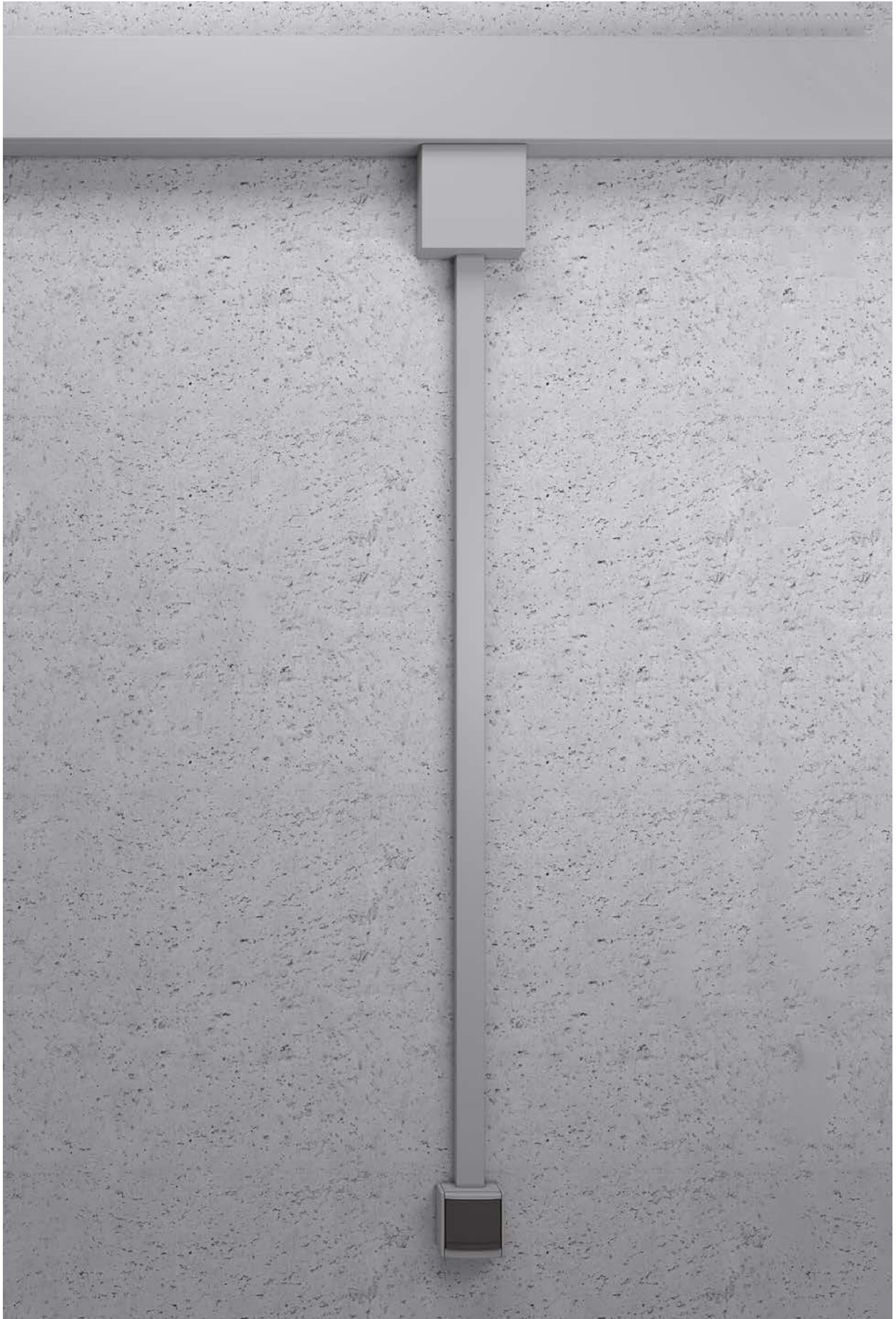
Industrial building: power supply
