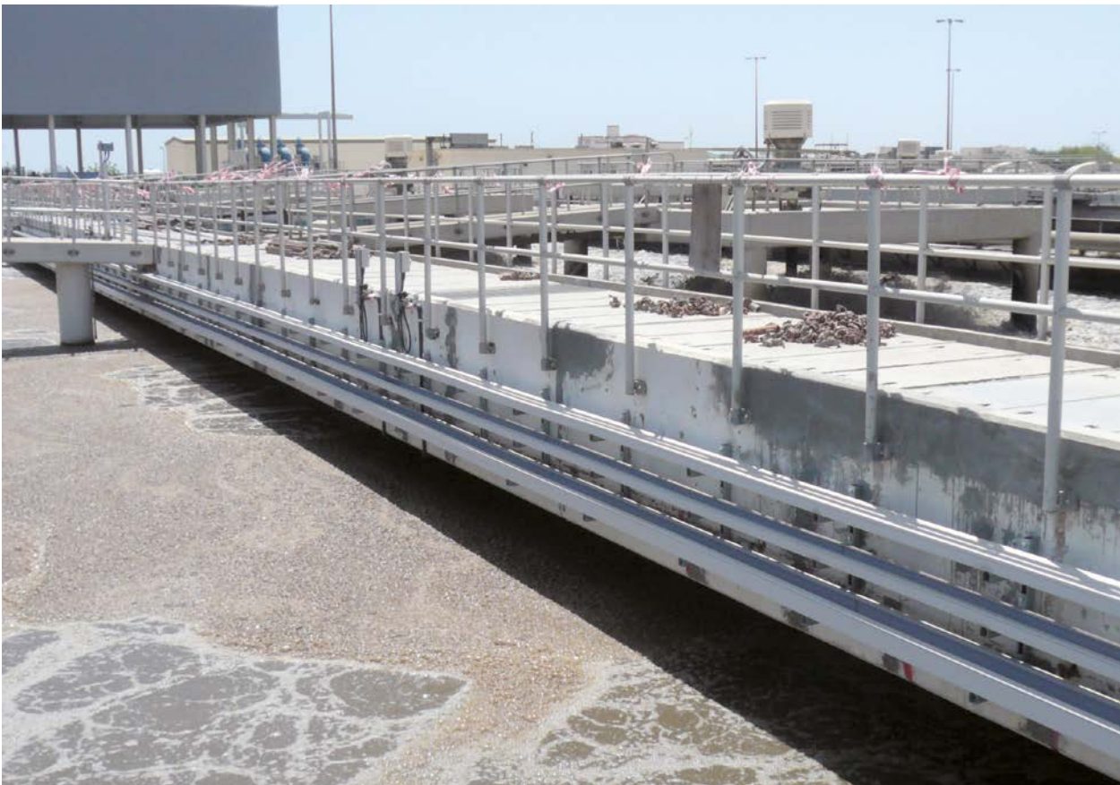
Waste water treatment plant
